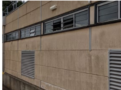
Figure 4: Example of RAAC in walls
