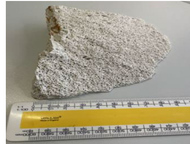
Figure 6: Aerated appearance of RAAC
