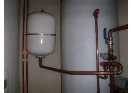
CYLINDER 2 EXPANSION VESSEL FIT FLUSHING VALVE FAULTY EXPANSION VESSEL
