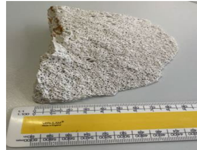
Figure 6: Aerated appearance of RAAC
