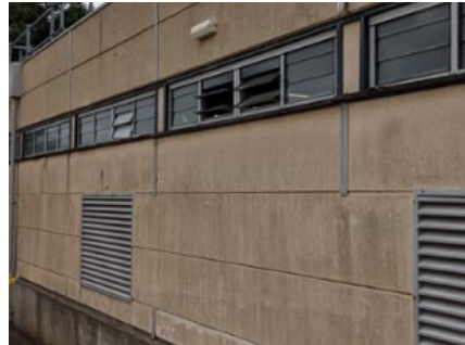
Figure 4: Example of RAAC in walls
