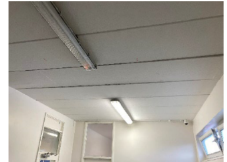
Figure 11: Example of deflected RAAC panel
