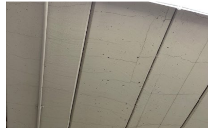
Figure 7: Underside of a cracked RAAC panel
