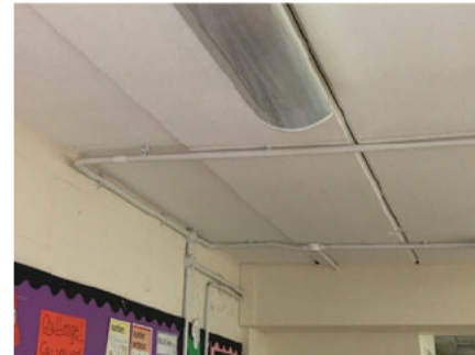
Figure 10: Example of deflected RAAC panel
