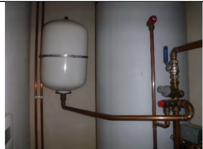
HWSV 02 FAULTY EXPANSION VESSEL
