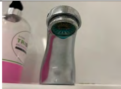
SLIGHT SCALE PRESENT ON OUTLETS
