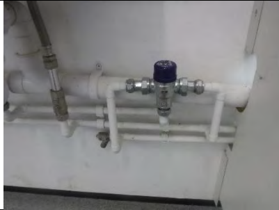
INSULATE MAINS PIPE WORK TMVS SERVICED 12/22
