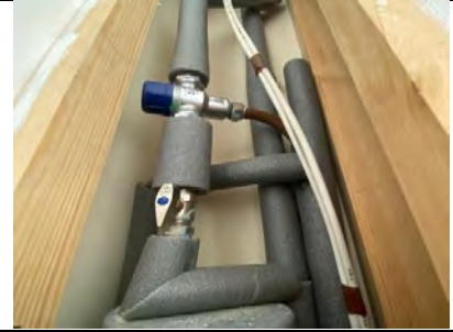
CENTRALISED TMV BEHIND THE PANEL IN DISABLED W/C
