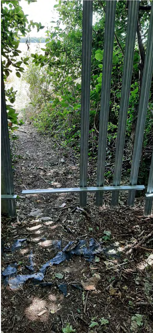
Damage to fences at Worcester Way
