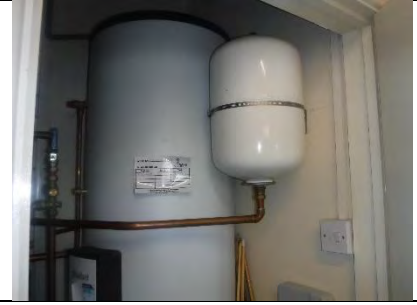
CYLINDER 1 EXPANSION VESSEL FIT FLUSHING VALVE
