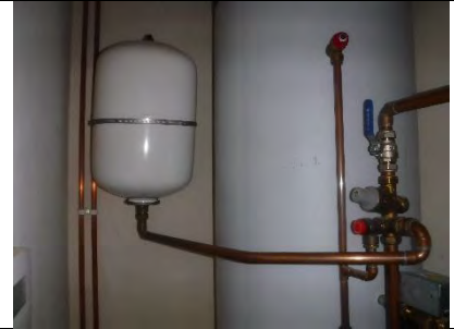
CYLINDER 2 EXPANSION VESSEL FIT FLUSHING VALVE FAULTY EXPANSION VESSEL
