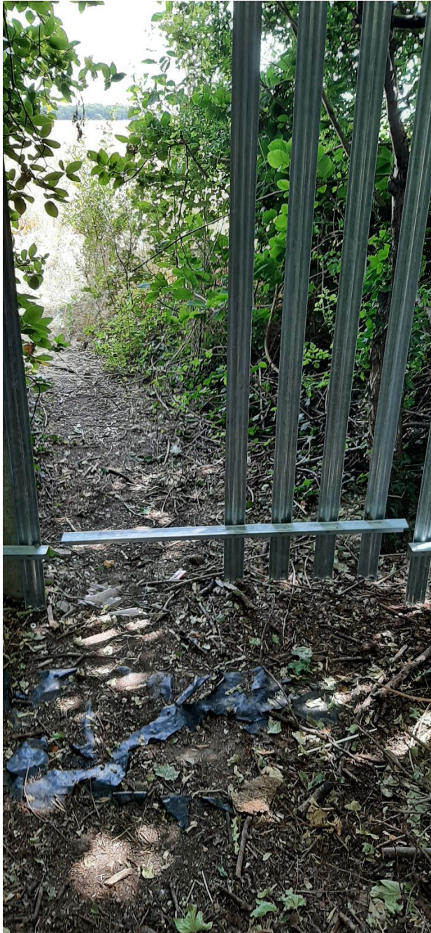
Damage to fences at Worcester Way
