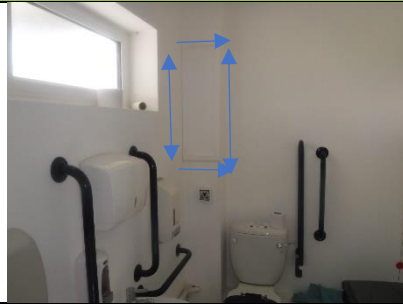
CENTRALISED TMV FITTED BEHIND PANEL IN DISABLED W/C
