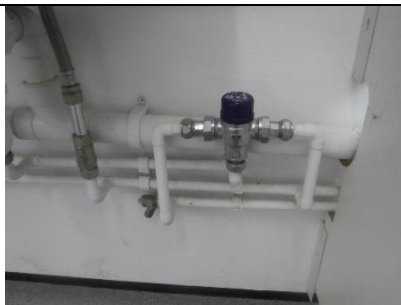
INSULATE MAINS PIPE WORK TMVS SERVICED 12/22
