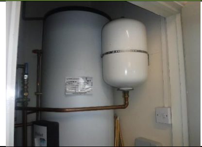
CYLINDER 1 EXPANSION VESSEL FIT FLUSHING VALVE
