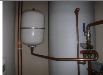
HWSV 02 FAULTY EXPANSION VESSEL
