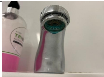
SLIGHT SCALE PRESENT ON OUTLETS
