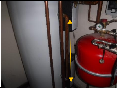
As there is no return pump existing pipework could be fitted with De-strat pumps so that luke warm water does not accumulate in the base of the water heaters
