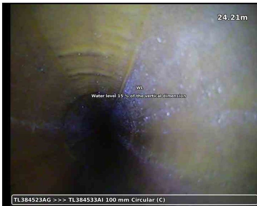
20210617-185600-snap0027.jpg, 00:05:54, 24.21 m Settled deposits, fine, 10% % cross-sectional area loss, S03
