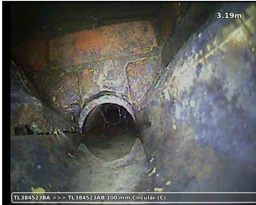
20210617-164942-snap0010.jpg, 00:01:45, 3.19 m Finish node type, manhole, reference number: TL384523AB
