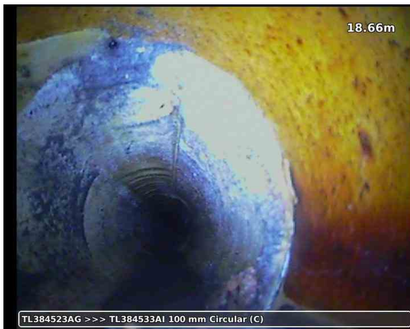
20210617-185600-snap0025.jpg, 00:04:58, 18.66 m Lining of drain or sewer with cured-in-place lining changes to polyester at this point
