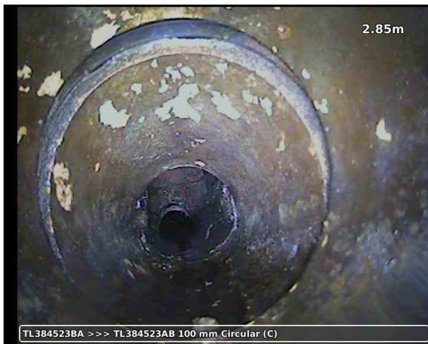
20210617-164942-snap0007.jpg, 00:01:15, 2.85 m Joint displaced, 10 mm displacement
