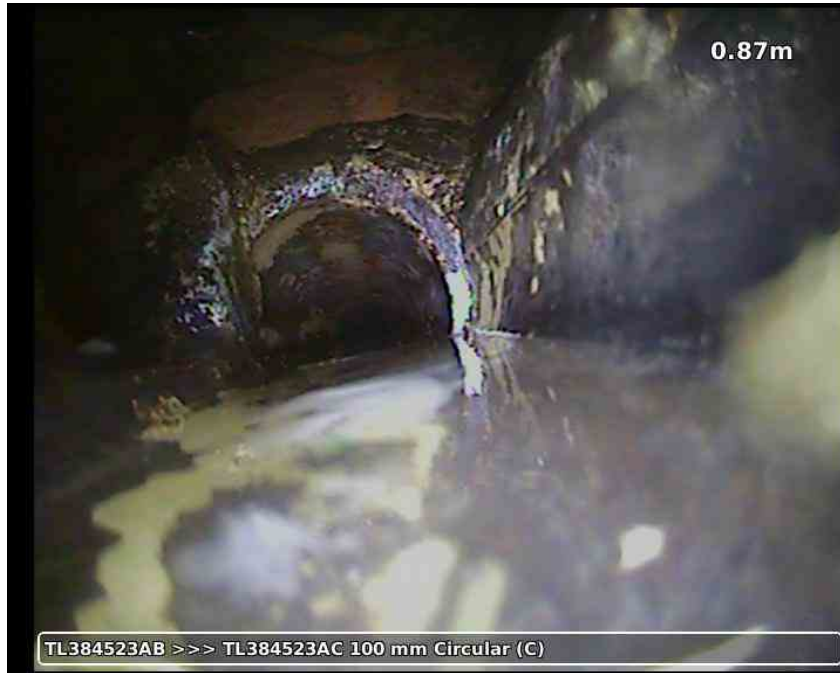
20210617-170147-snap0004.jpg, 00:00:43, 0.87 m Finish node type, manhole, reference number: TL384523AC
