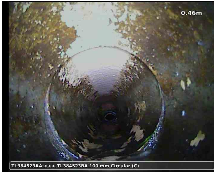
20210617-163005-snap0004.jpg, 00:00:39, 0.46 m Joint displaced, medium
