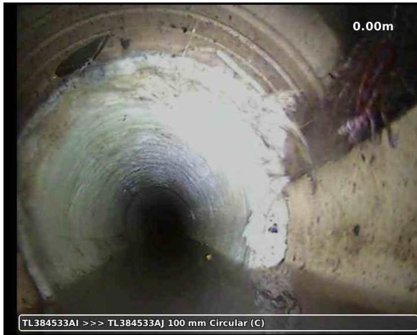
20210617-191337-snap0002.jpg, 00:00:19, 0.00 m Lining of drain or sewer with cured-in-place lining changes to epoxy at this point
