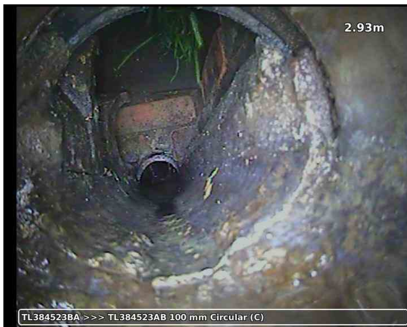
20210617-164942-snap0009.jpg, 00:01:35, 2.93 m Settled deposits, hard or compacted, 20% % cross-sectional area loss
