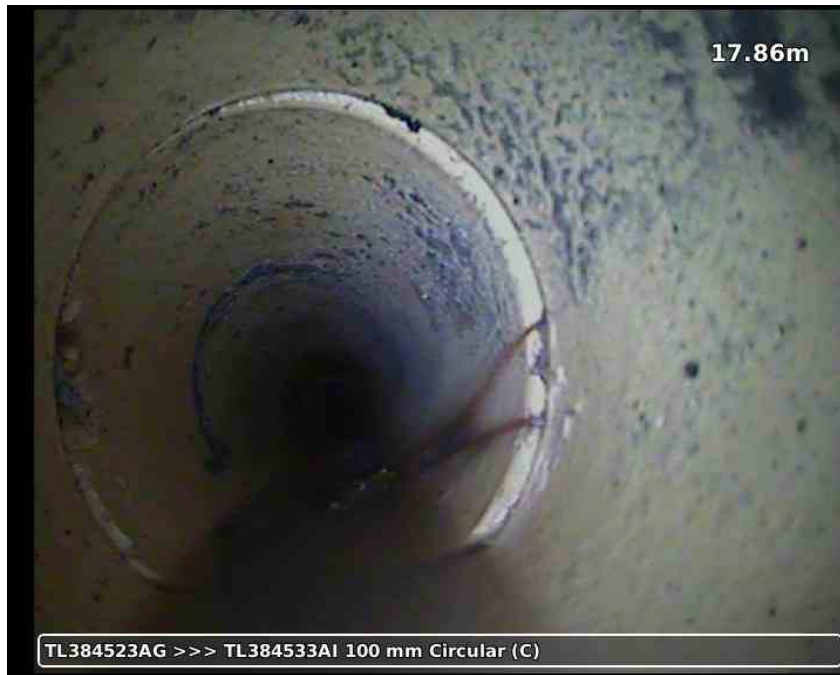
20210617-185600-snap0020.jpg, 00:04:16, 17.86 m Roots, fine at joint
