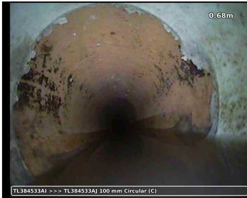
20210617-191337-snap0004.jpg, 00:00:56, 0.68 m Cured-in-place lining ends at this point
