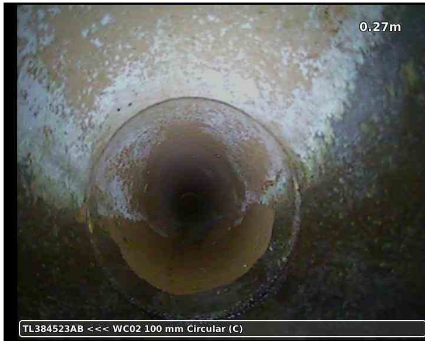
20210617-165855-snap0002.jpg, 00:00:15, 0.27 m Attached deposits, fouling, from 02 to 10 o'clock, 5% % cross-sectional area loss
