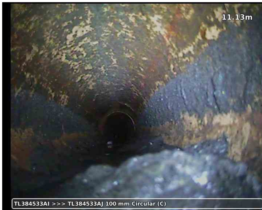
20210617-191337-snap0013.jpg, 00:03:52, 11.13 m Settled deposits, fine, 20% % cross-sectional area loss, S03
