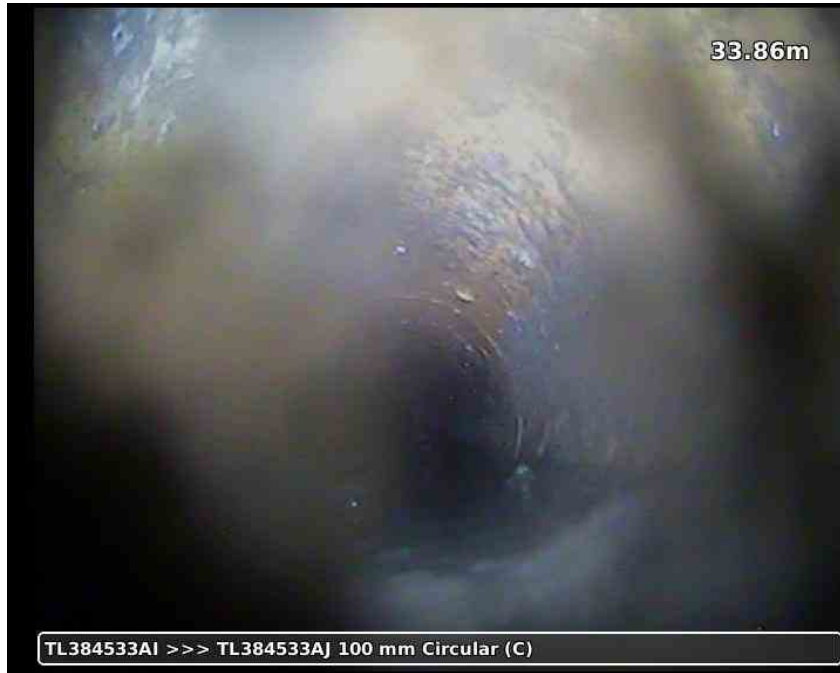
20210617-191337-snap0024.jpg, 00:08:16, 33.86 m Settled deposits, fine, 30% % cross-sectional area loss, S08
