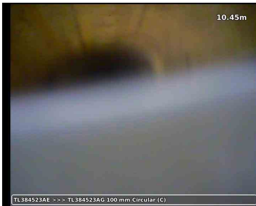
20210617-181934-snap0007.jpg, 00:02:12, 10.45 m Loss of vision, camera under water, S01
