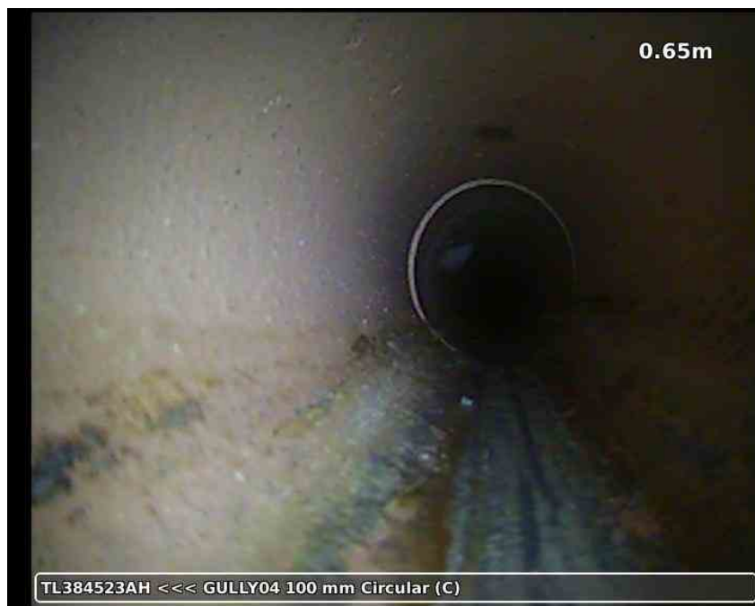
20210617-183231-snap0003.jpg, 00:00:12, 0.65 m Attached deposits, encrustation, from 05 to 07 o'clock, 5% % cross-sectional area loss, S01, Scale
