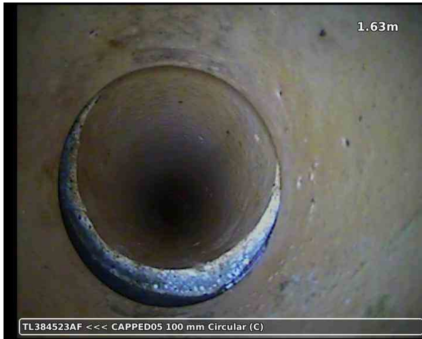
20210617-180419-snap0002.jpg, 00:00:34, 1.63 m Joint displaced, 10 mm displacement
