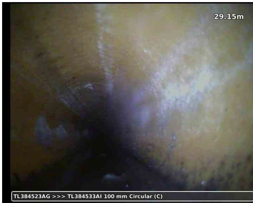
20210617-185600-snap0031.jpg, 00:06:58, 29.15 m Settled deposits, fine, 20% % cross-sectional area loss, S05
