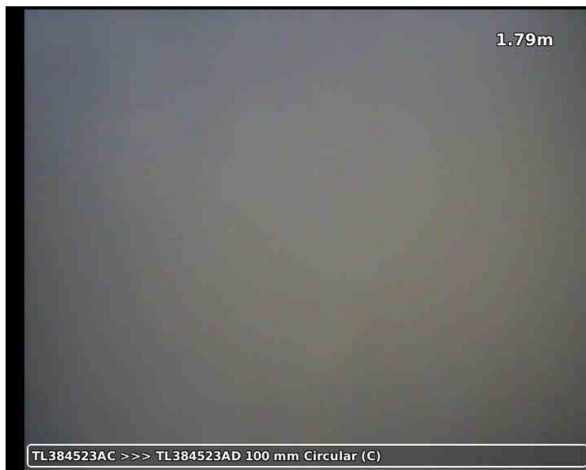
20210617-171630-snap0005.jpg, 00:01:19, 1.79 m Lining of drain or sewer with cured-in-place lining changes to polyester at this point
