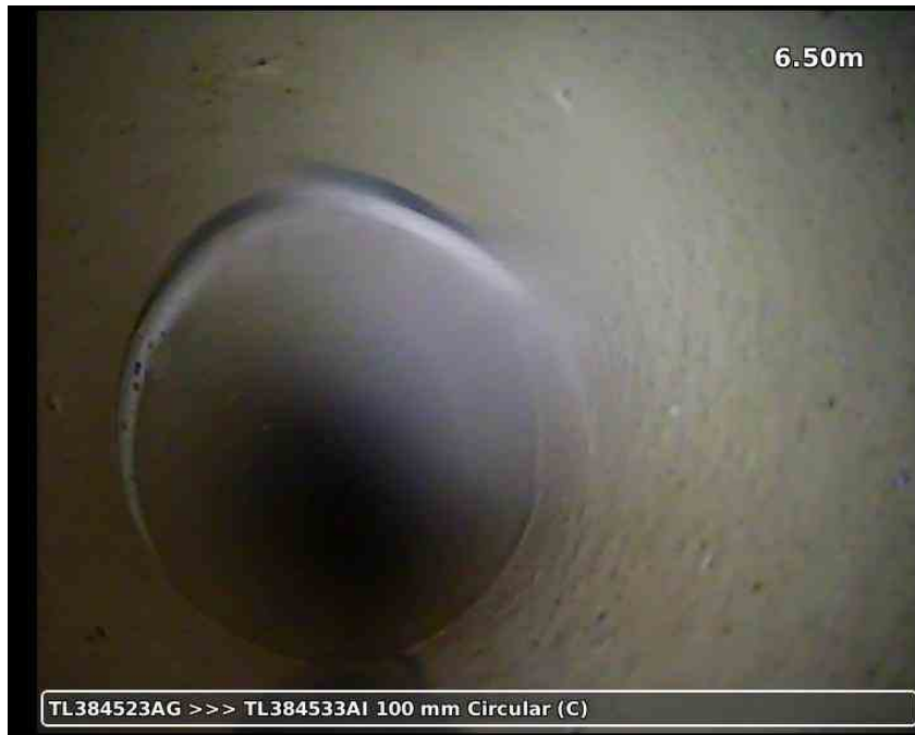
20210617-185600-snap0010.jpg, 00:02:16, 6.50 m Joint displaced, medium
