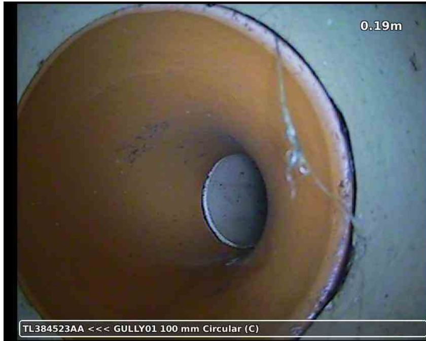
20210617-161336-snap0002.jpg, 00:00:11, 0.19 m Roots, fine at joint
