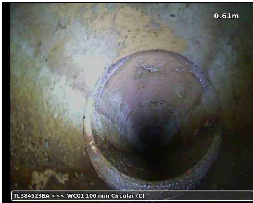
20210617-164432-snap0006.jpg, 00:00:45, 0.61 m Joint displaced, 10 mm displacement
