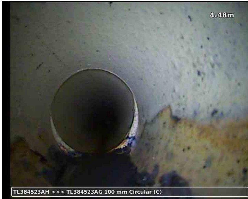
20210617-184209-snap0002.jpg, 00:00:40, 4.48 m Settled deposits, fine at joint, 15% % cross-sectional area loss
