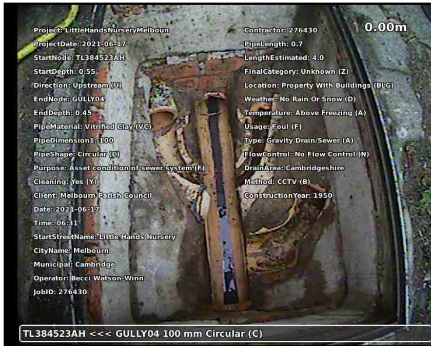
20210617-183231-snap0000.jpg, 00:00:00, 0.00 m Start node type, manhole, reference number: TL384523AH
