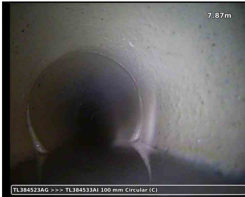
20210617-185600-snap0012.jpg, 00:02:36, 7.87 m Joint displaced, medium
