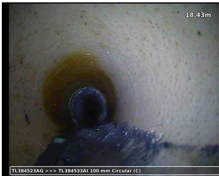
20210617-185600-snap0023.jpg, 00:04:41, 18.43 m Crack, circumferential, from 07 to 05 o'clock
