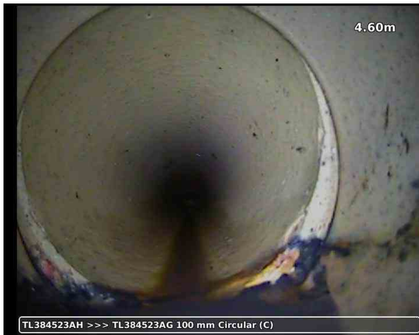
20210617-184209-snap0003.jpg, 00:00:53, 4.60 m Joint displaced, medium
