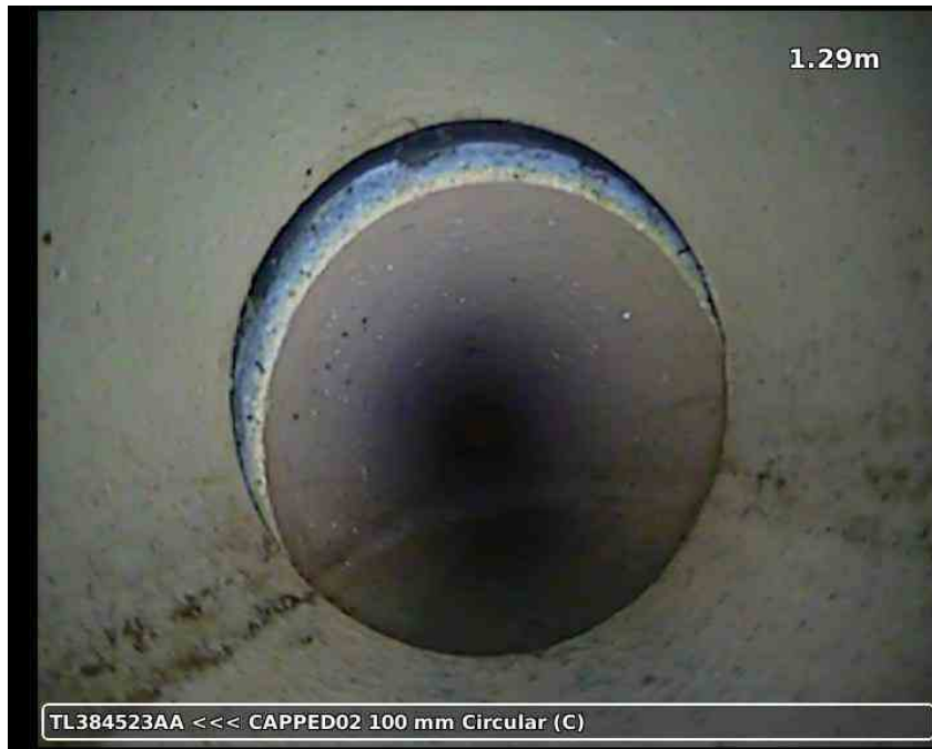
20210617-161854-snap0002.jpg, 00:00:28, 1.29 m Joint displaced, 10 mm displacement
