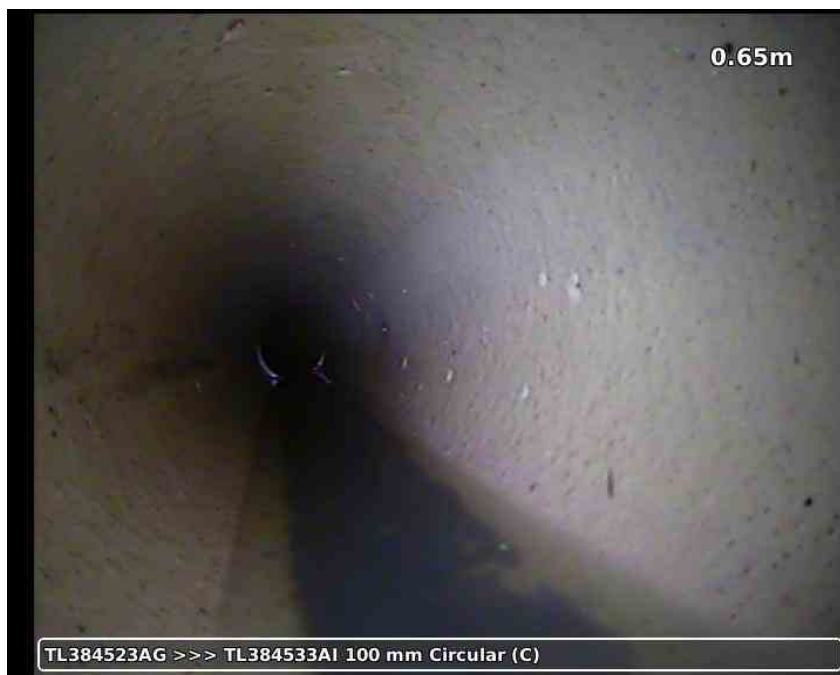
20210617-185600-snap0003.jpg, 00:00:19, 0.65 m Settled deposits, fine, 5% % cross-sectional area loss, S01
