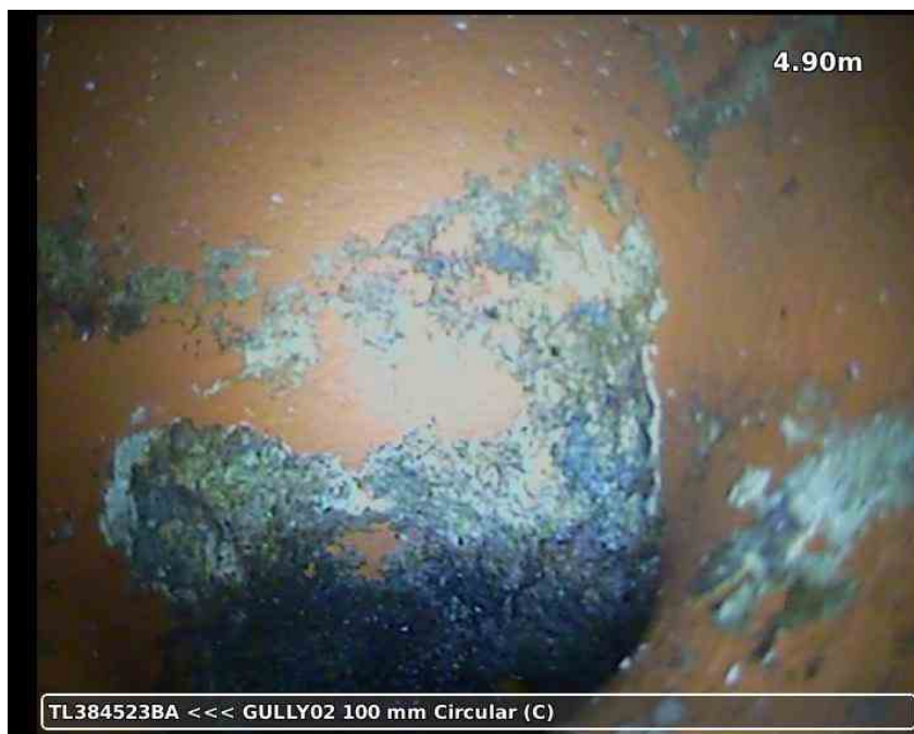
20210617-164707-snap0005.jpg, 00:01:19, 4.90 m Finish node type, gully, reference number: GULLY02, DISUSED INTERNAL GULLY
