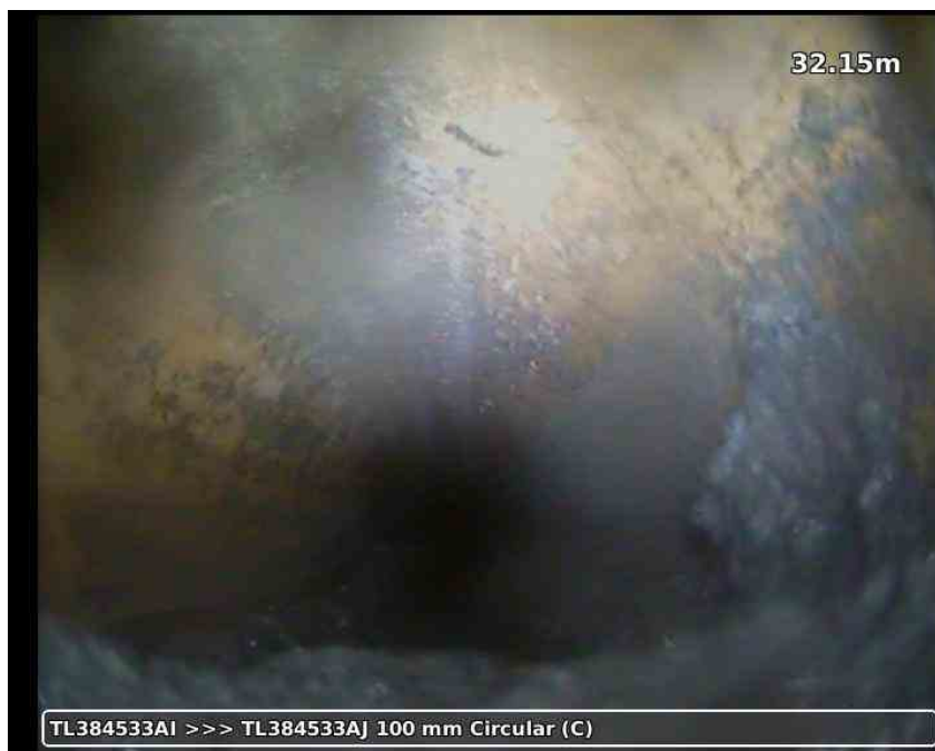
20210617-191337-snap0023.jpg, 00:07:53, 32.15 m Settled deposits, fine, 20% % cross-sectional area loss, S07
