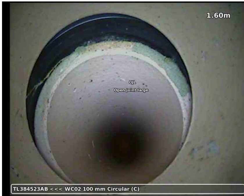
20210617-165855-snap0004.jpg, 00:00:40, 1.60 m Joint displaced, 20 mm displacement
