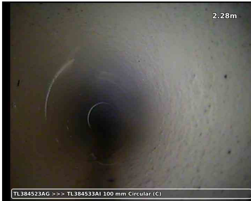
20210617-185600-snap0006.jpg, 00:01:02, 2.28 m Fracture, longitudinal, at 11 o'clock
