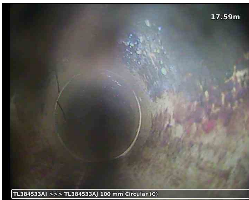
20210617-191337-snap0015.jpg, 00:05:00, 17.59 m Roots, fine at joint
