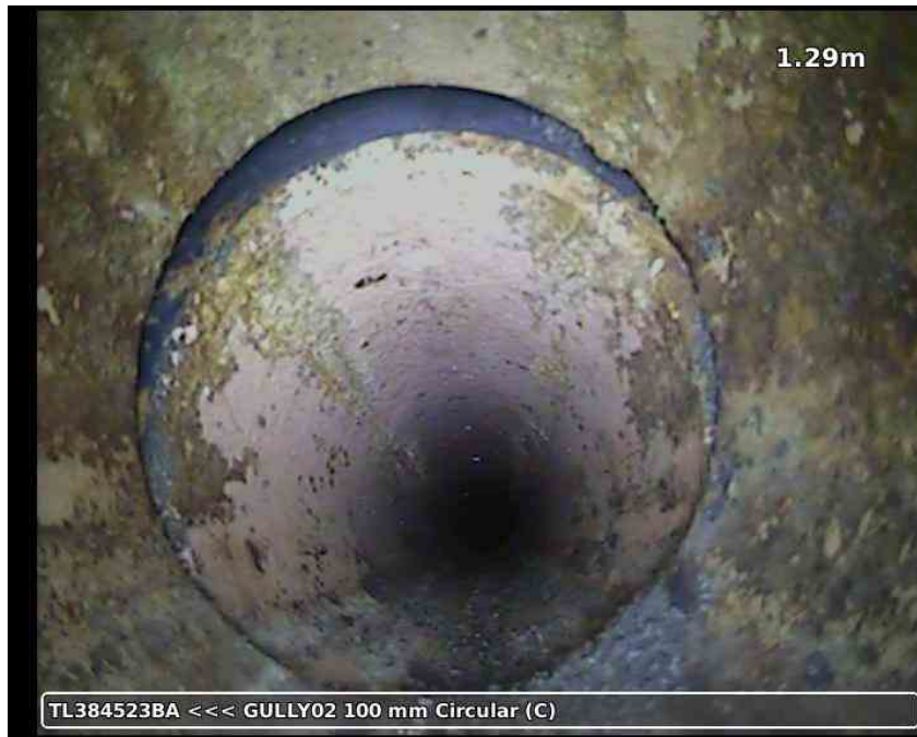
20210617-164707-snap0004.jpg, 00:00:39, 1.29 m Joint displaced, 10 mm displacement
