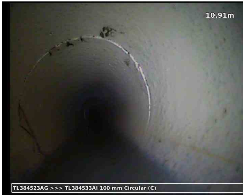
20210617-185600-snap0016.jpg, 00:03:14, 10.91 m Fracture, circumferential, from 07 to 05 o'clock
