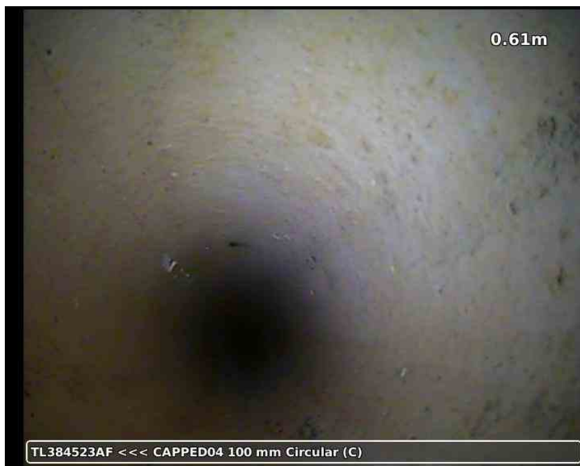
20210617-180144-snap0003.jpg, 00:00:35, 0.61 m Fracture, longitudinal, at 11 o'clock, S01
