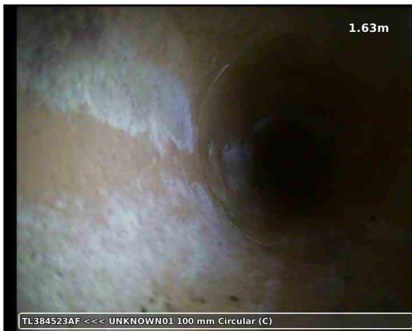
20210617-175837-snap0003.jpg, 00:00:41, 1.63 m Fracture, circumferential, from 03 to 11 o'clock
