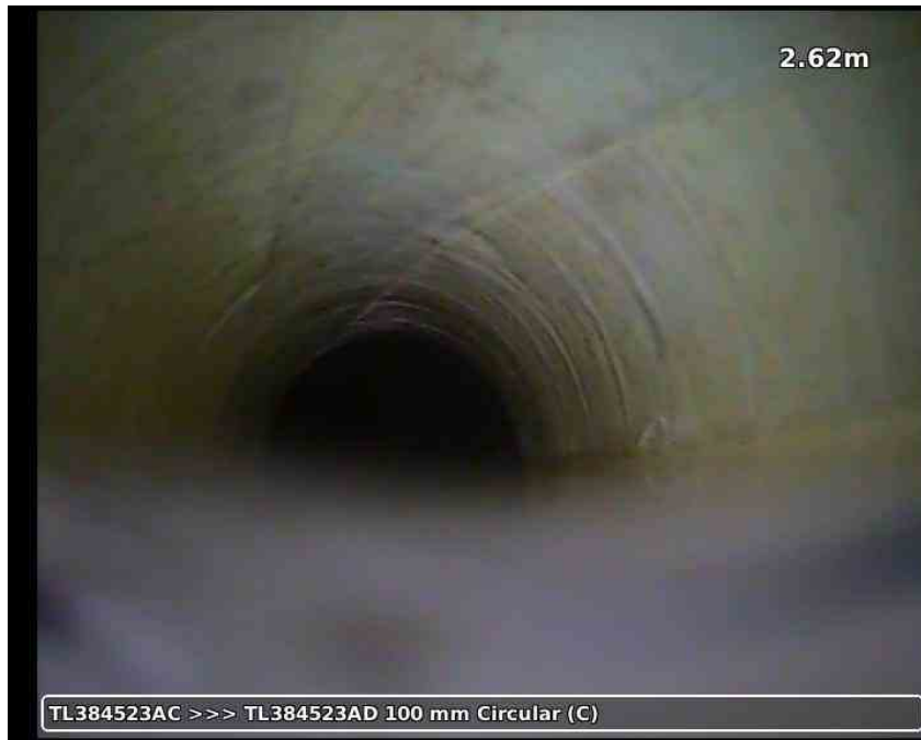
20210617-171630-snap0007.jpg, 00:02:01, 2.62 m Cured-in-place lining ends at this point
