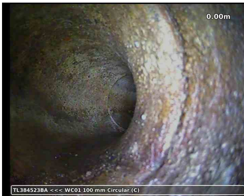
20210617-164432-snap0003.jpg, 00:00:15, 0.00 m Attached deposits, fouling, from 01 to 12 o'clock, 5% % cross-sectional area loss, S01
