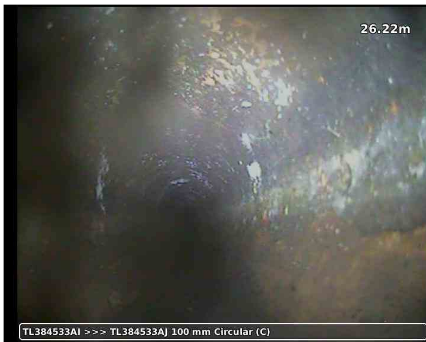
20210617-191337-snap0019.jpg, 00:06:24, 26.22 m Settled deposits, fine, 10% % cross-sectional area loss, S05
