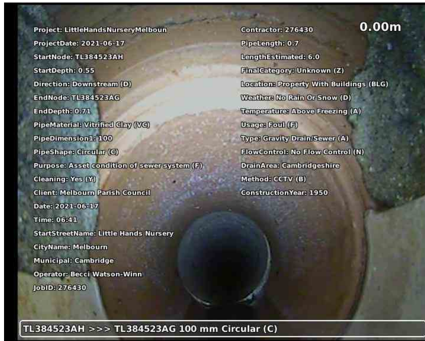
20210617-184209-snap0000.jpg, 00:00:01, 0.00 m Start node type, manhole, reference number: TL384523AH
