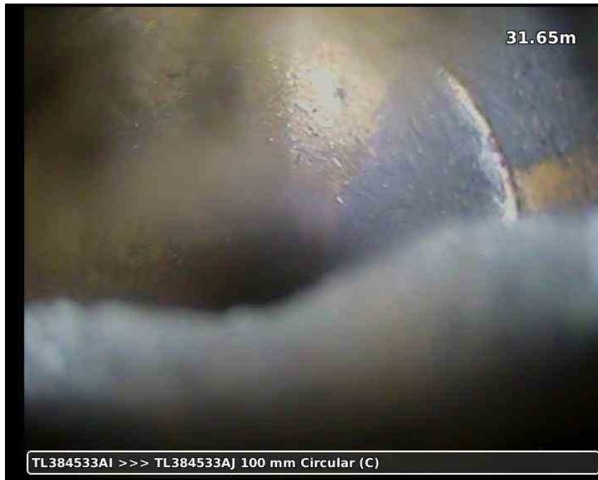
20210617-191337-snap0022.jpg, 00:07:42, 31.65 m Settled deposits, fine, 30% % cross-sectional area loss
