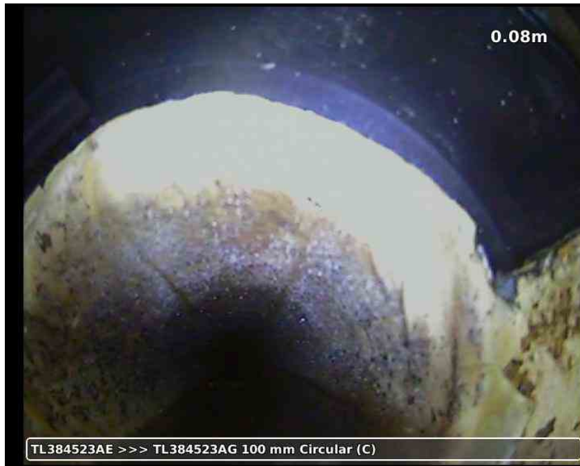
20210617-181934-snap0002.jpg, 00:00:16, 0.08 m Lining of drain or sewer with cured-in-place lining changes to polyester at this point
