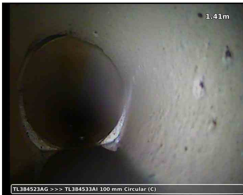
20210617-185600-snap0005.jpg, 00:00:45, 1.41 m Joint displaced, medium
