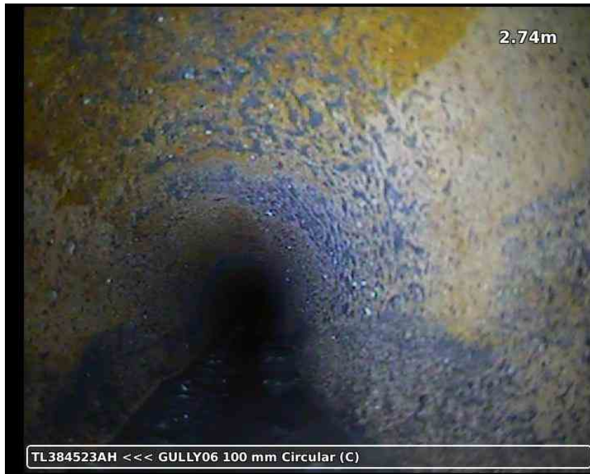
20210617-183738-snap0004.jpg, 00:00:52, 2.74 m Settled deposits, fine, 10% % cross-sectional area loss, S02
