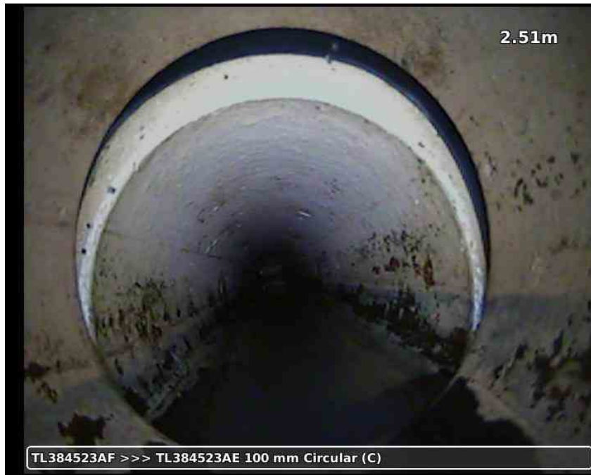
20210617-180721-snap0002.jpg, 00:00:46, 2.51 m Joint displaced, 20 mm displacement
