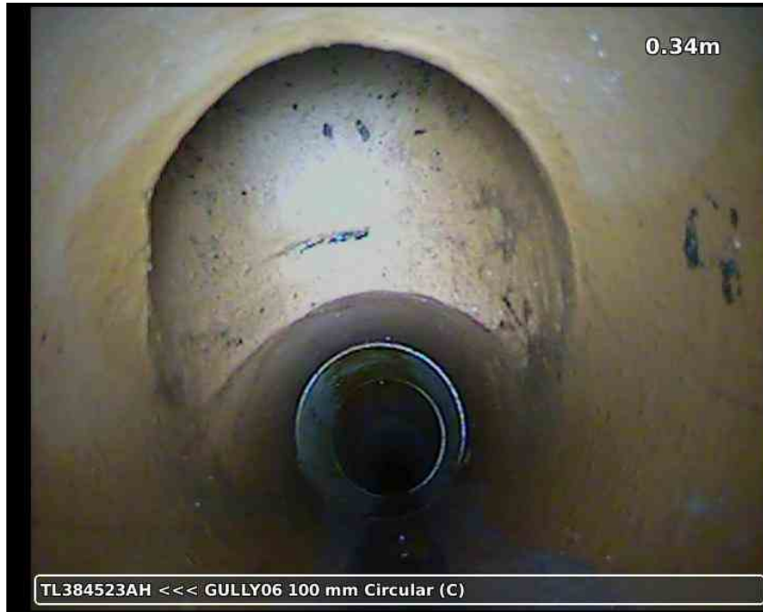
20210617-183738-snap0002.jpg, 00:00:12, 0.34 m Junction, at 12 o'clock, diameter: 100 mm, UNKNOWN CONNECTION
