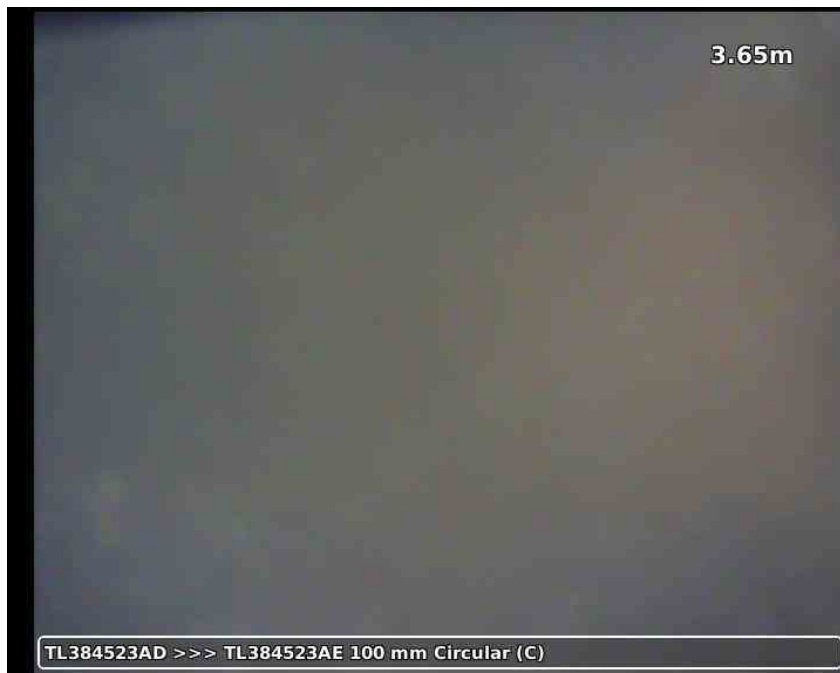
20210617-173215-snap0005.jpg, 00:01:34, 3.65 m Loss of vision, camera under water, S01
