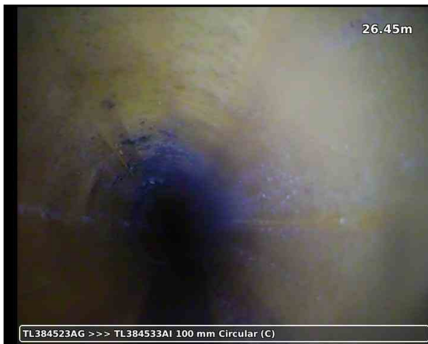
20210617-185600-snap0029.jpg, 00:06:26, 26.41 m Settled deposits, fine, 5% % cross-sectional area loss, S04
