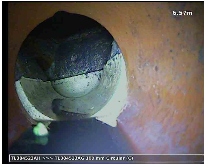
20210617-184209-snap0006.jpg, 00:01:30, 6.57 m Joint displaced, 10 mm displacement
