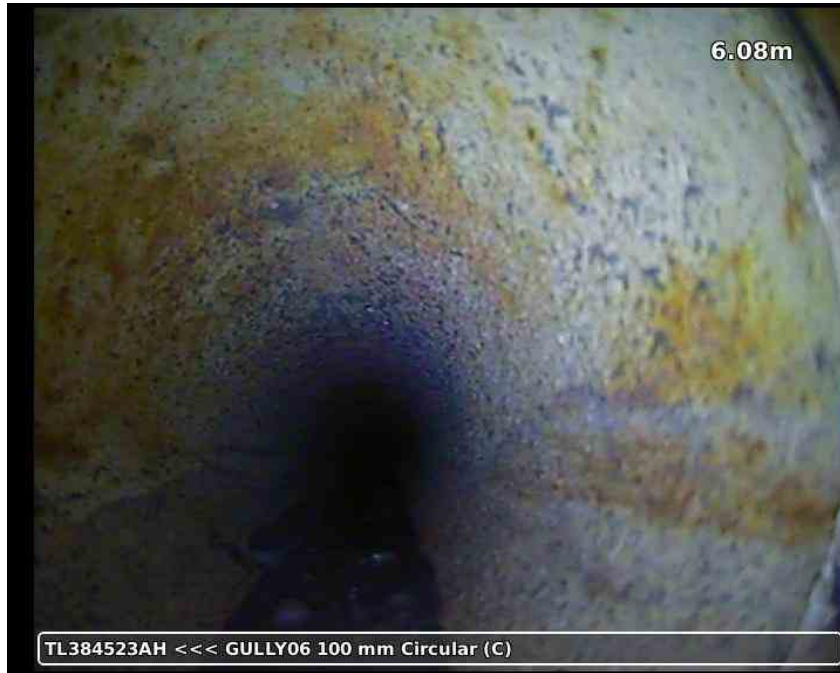
20210617-183738-snap0006.jpg, 00:01:33, 6.08 m Settled deposits, fine, 10% % cross-sectional area loss, S04
