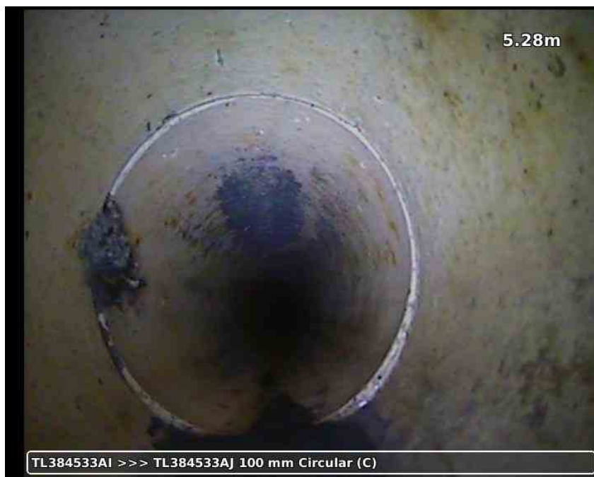
20210617-191337-snap0007.jpg, 00:01:58, 5.28 m Roots, mass at joint, 5% % cross-sectional area loss
