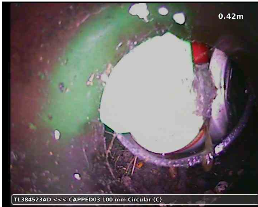
20210617-172705-snap0002.jpg, 00:00:31, 0.42 m General remark, APPEARS TO BE A CAPPED OFF LINE
