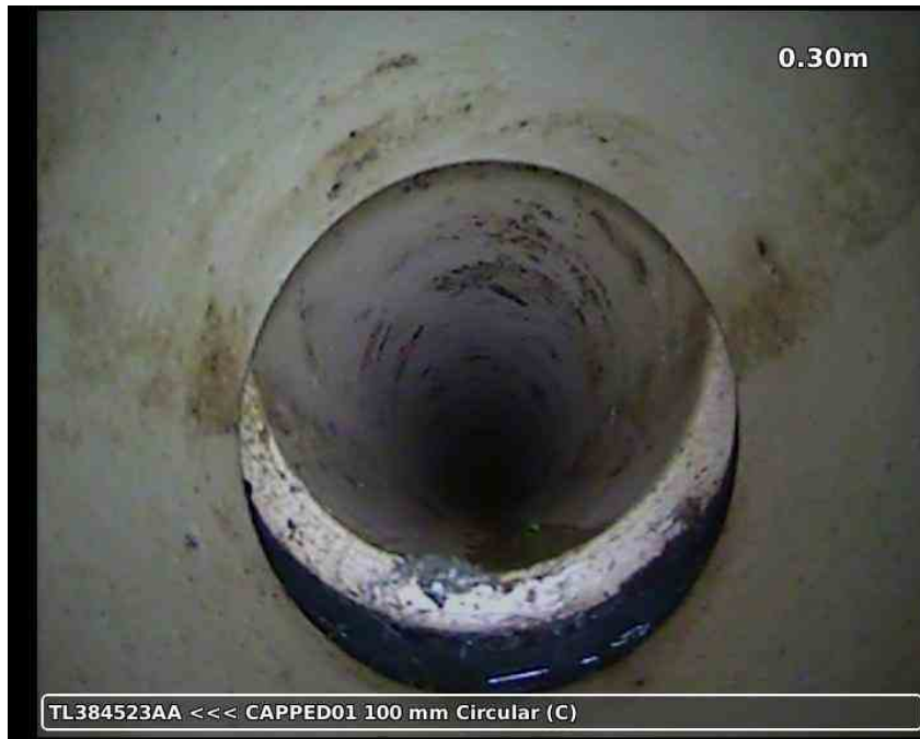
20210617-161651-snap0002.jpg, 00:00:18, 0.30 m Joint displaced, 20 mm displacement
