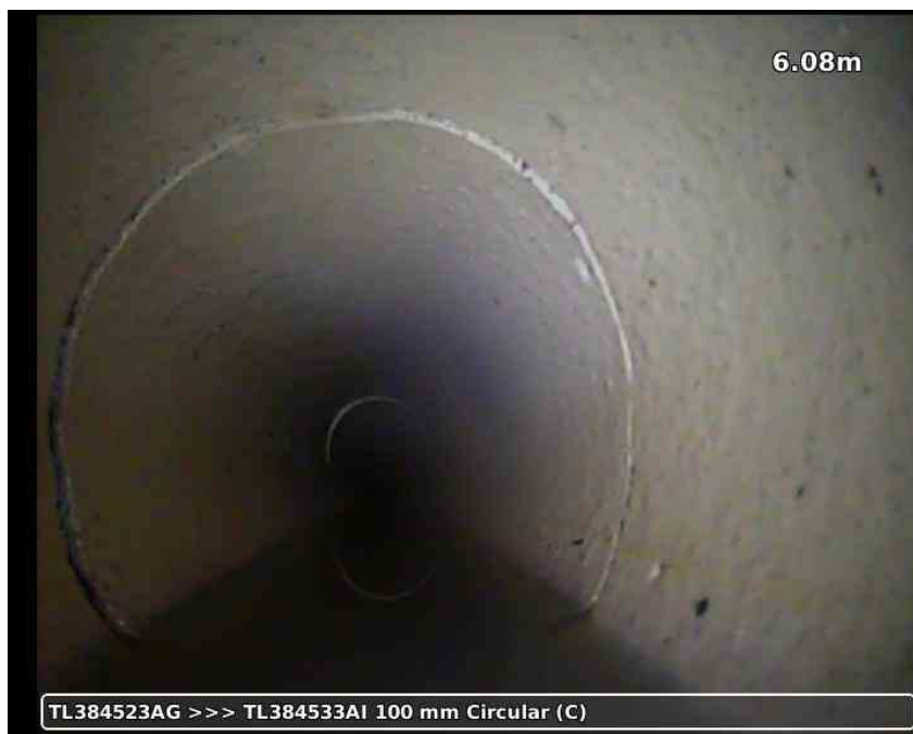
20210617-185600-snap0009.jpg, 00:02:01, 6.08 m Fracture, circumferential, from 07 to 05 o'clock
