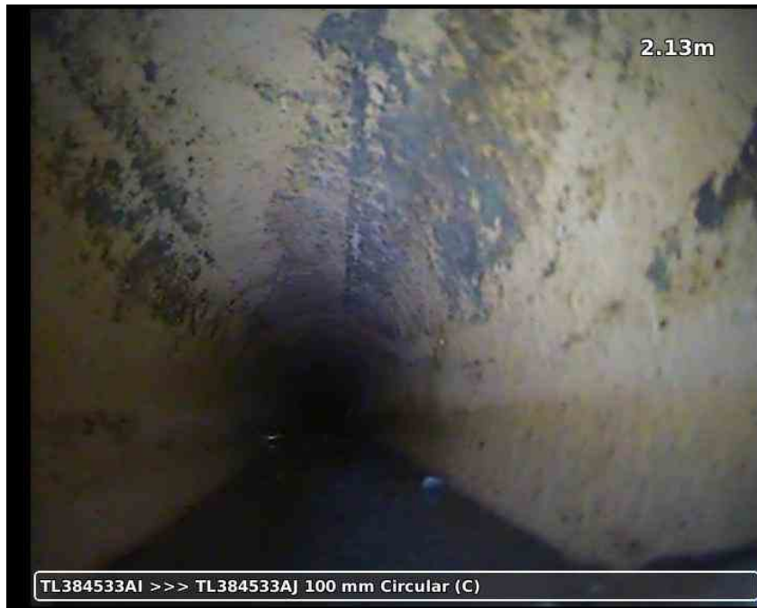
20210617-191337-snap0006.jpg, 00:01:20, 2.13 m Settled deposits, fine, 10% % cross-sectional area loss, S01
