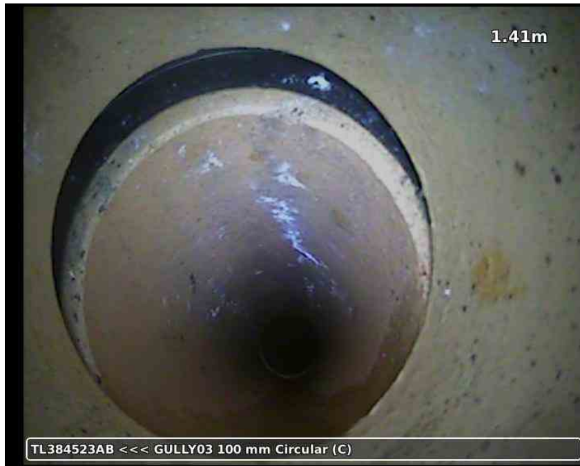
20210617-165624-snap0002.jpg, 00:00:24, 1.41 m Joint displaced, 20 mm displacement
