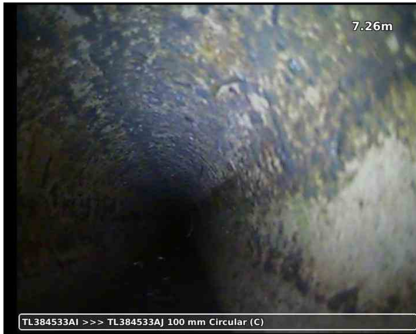
20210617-191337-snap0010.jpg, 00:02:38, 7.26 m Attached deposits, fouling, from 07 to 05 o'clock, 5% % cross-sectional area loss, S02
