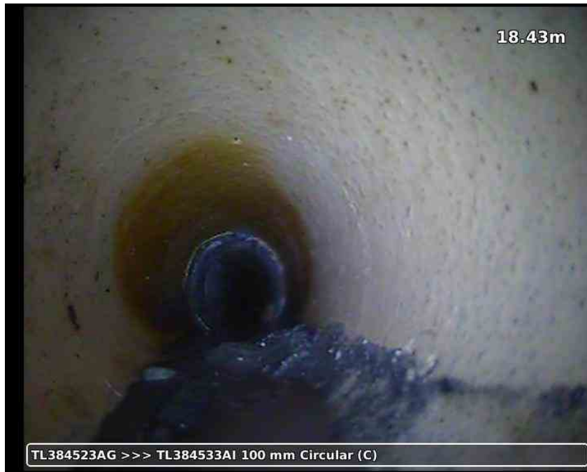
20210617-185600-snap0024.jpg, 00:04:45, 18.43 m Settled deposits, fine, 10% % cross-sectional area loss, S02
