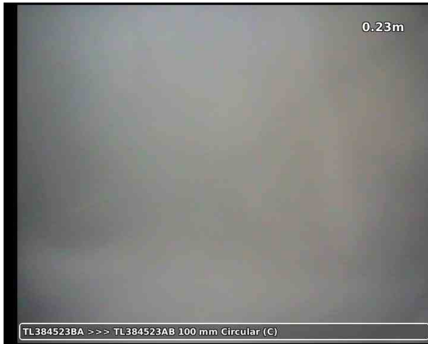
20210617-164942-snap0002.jpg, 00:00:14, 0.23 m Loss of vision, camera under water, S01
