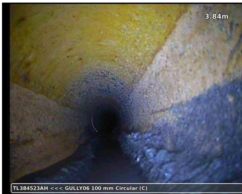
20210617-183738-snap0005.jpg, 00:01:13, 3.84 m Settled deposits, fine, 20% % cross-sectional area loss, S03
