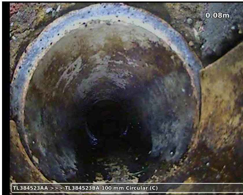
20210617-163005-snap0002.jpg, 00:00:17, 0.08 m Joint displaced, medium
