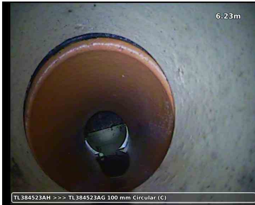
20210617-184209-snap0004.jpg, 00:01:12, 6.23 m Joint displaced, medium
