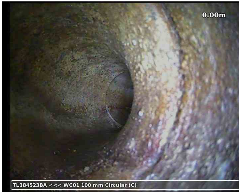
20210617-164432-snap0002.jpg, 00:00:09, 0.00 m General remark, LINE HASN'T BEEN CLEANED PRE SURVEY
