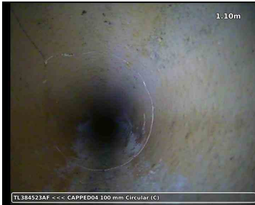
20210617-180144-snap0004.jpg, 00:00:50, 1.10 m Fracture, circumferential, from 11 to 10 o'clock
