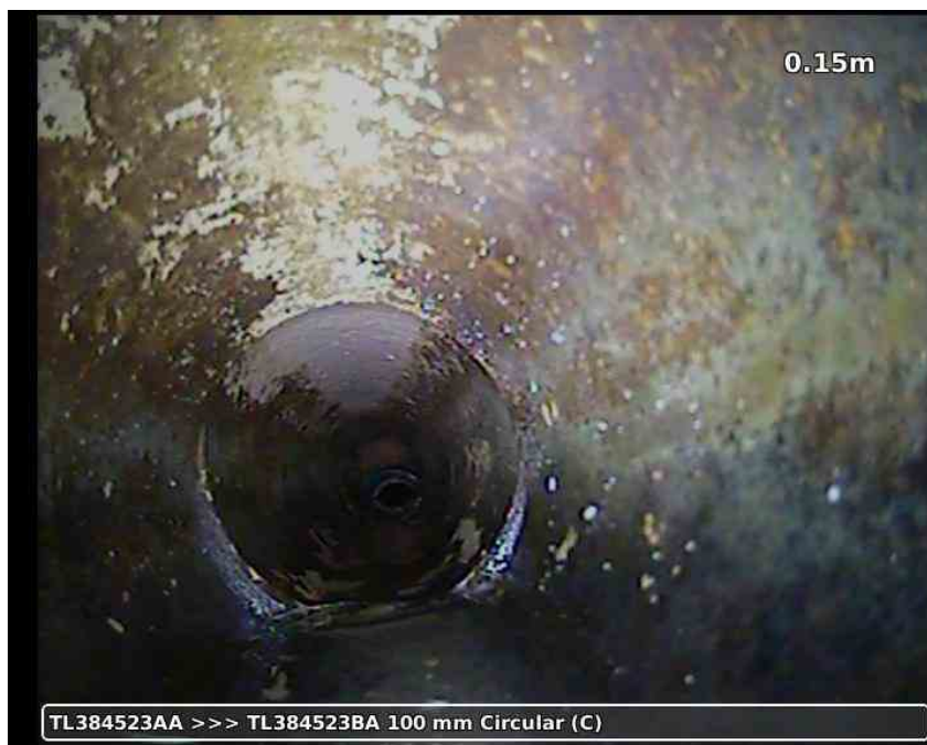
20210617-163005-snap0003.jpg, 00:00:25, 0.15 m Attached deposits, fouling, from 01 to 11 o'clock, 5% % cross-sectional area loss, S01
