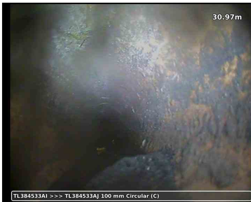
20210617-191337-snap0021.jpg, 00:07:19, 30.97 m Settled deposits, fine, 10% % cross-sectional area loss, S06
