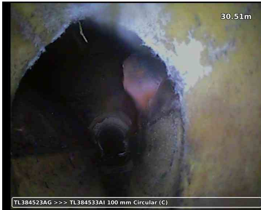
20210617-185600-snap0032.jpg, 00:07:27, 30.51 m Cured-in-place lining ends at this point
