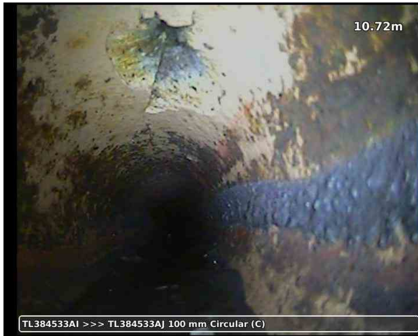
20210617-191337-snap0012.jpg, 00:03:34, 10.72 m Hole in drain or sewer, from 11 to 01 o'clock
