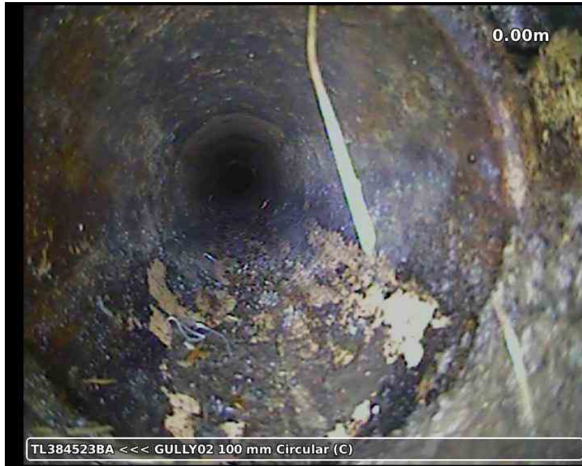
20210617-164707-snap0002.jpg, 00:00:12, 0.00 m Attached deposits, fouling, from 01 to 12 o'clock, 5% % cross-sectional area loss, S01
