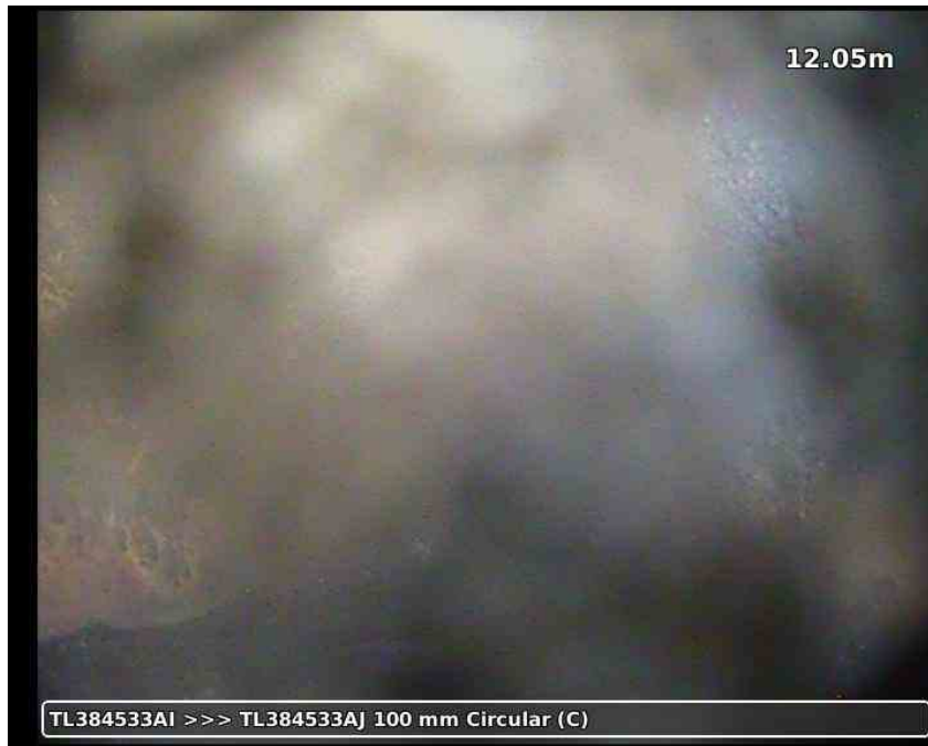
20210617-191337-snap0014.jpg, 00:04:06, 12.05 m Loss of vision, silt, S04
