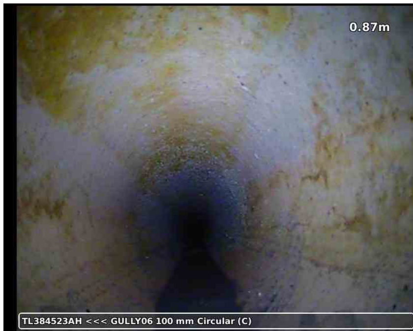
20210617-183738-snap0003.jpg, 00:00:29, 0.87 m Settled deposits, fine, 10% % cross-sectional area loss, S01
