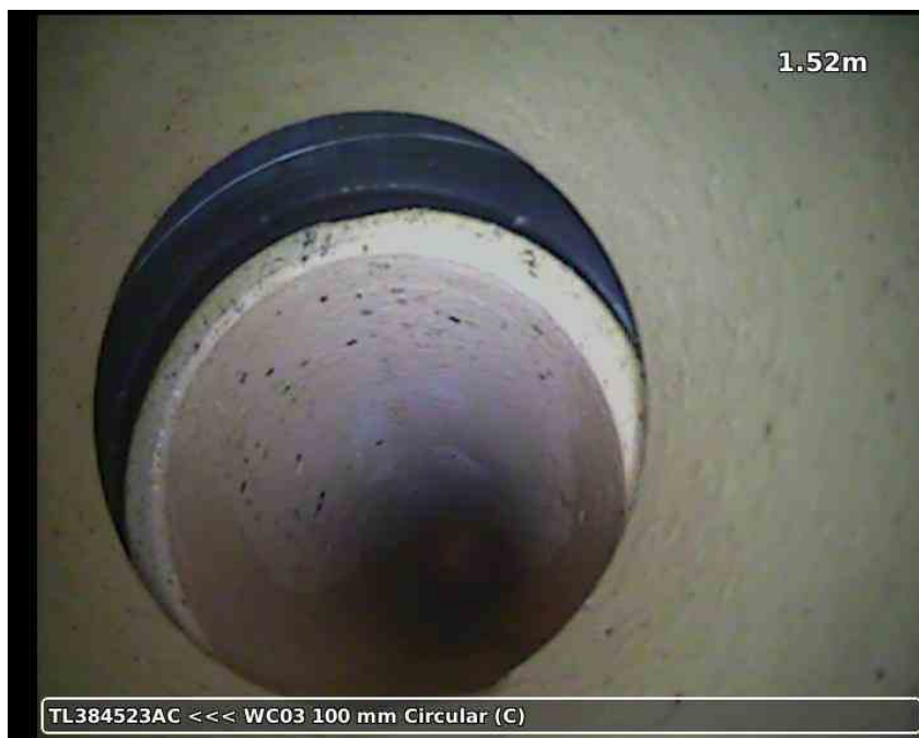
20210617-171046-snap0003.jpg, 00:00:27, 1.52 m Joint displaced, 20 mm displacement
