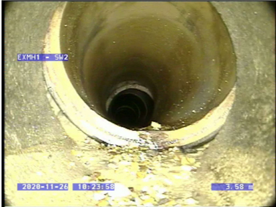
Photo: 5_5_26_A.jpg 3.7m, Joint displaced, medium
