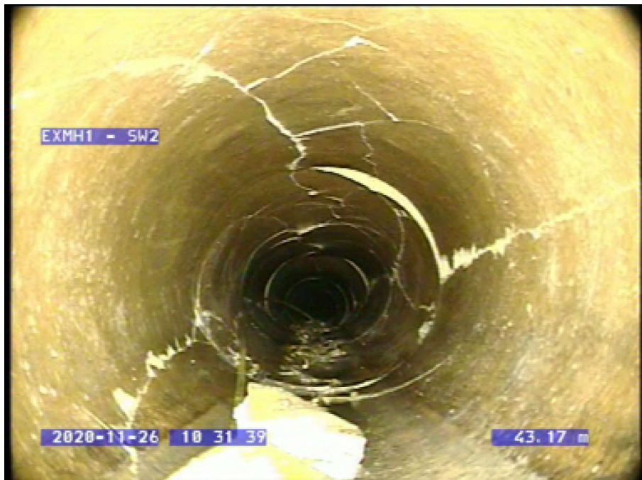
Photo: 5_5_50_A.jpg 43.2m, Fracture, multiple, from 12 to 12 o'clock, Start
