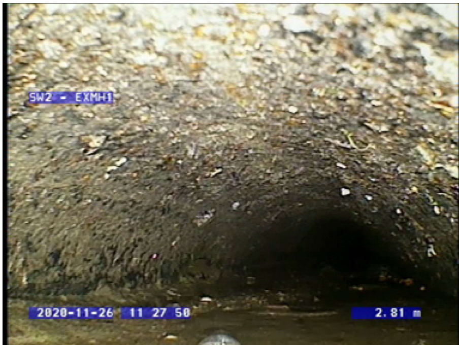
Photo: 7_7_69_A.jpg 3m, Settled deposits, coarse, 50% cross-sectional area loss, End
