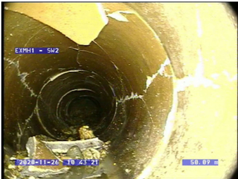
Photo: 5_5_55_A.jpg 50.1m, Broken pipe, from 12 to 12 o'clock, End
