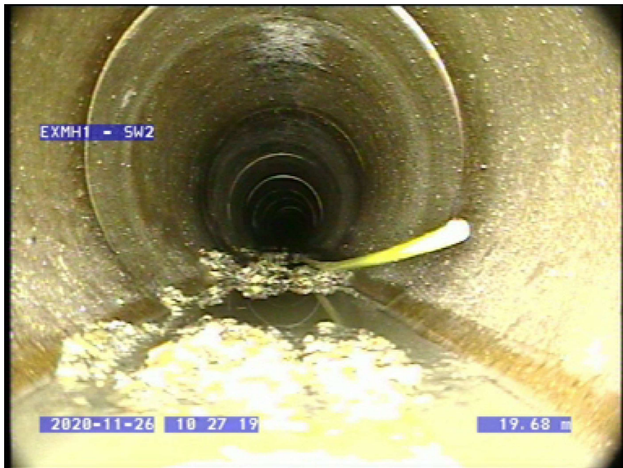
Photo: 5_5_36_A.jpg 19.8m, Other obstacles, external pipe or cable, at 5 o'clock, 5% cross-sectional area loss, Start
