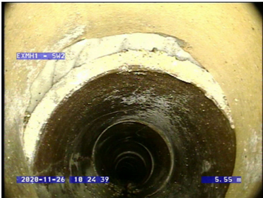
Photo: 5_5_28_A.jpg 5m, Joint displaced, medium
