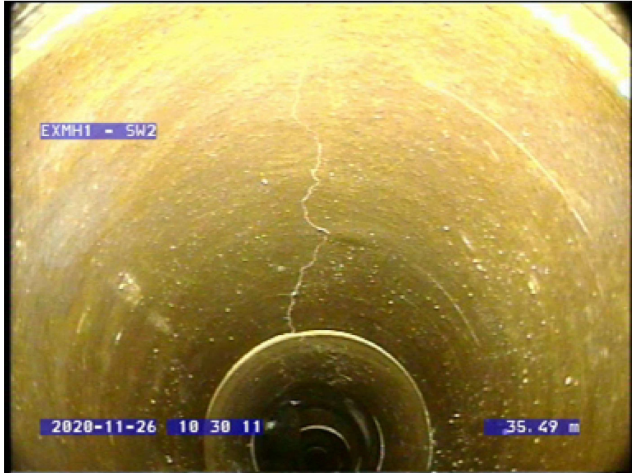
Photo: 5_5_40_A.jpg 35.5m, Crack, longitudinal at joint, at 12 o'clock
