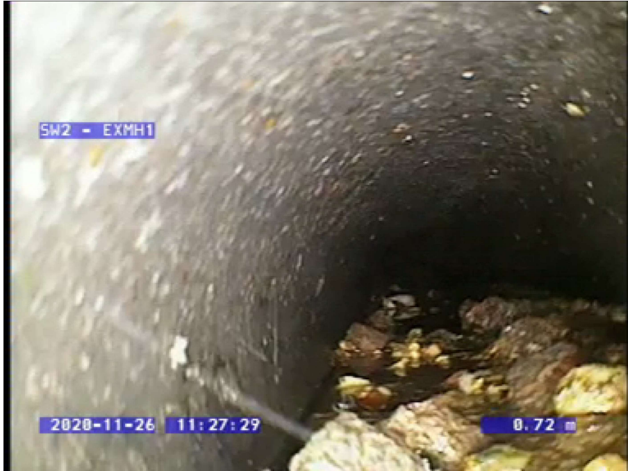
Photo: 7_7_64_A.jpg 0.5m, Settled deposits, coarse, 50% cross-sectional area loss, Start
