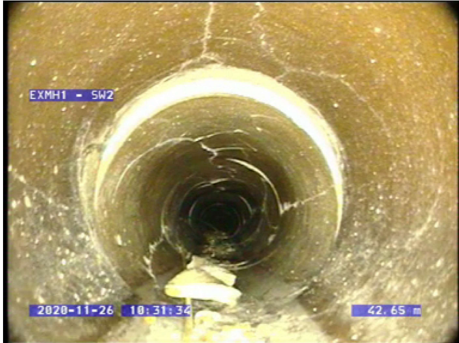
Photo: 5_5_48_A.jpg 42.7m, Cracks, multiple, from 12 to 12 o'clock, End
