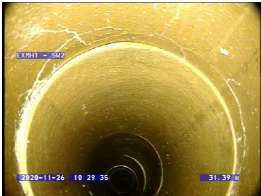
Photo: 5_5_39_A.jpg 31.4m, Crack, circumferential at joint, from 10 to 3 o'clock
