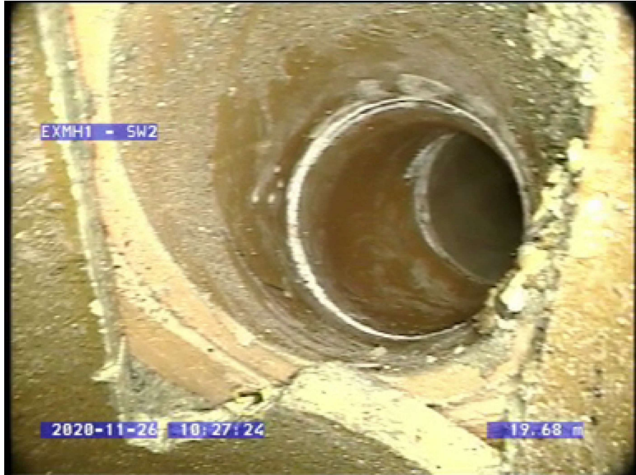
Photo: 5_5_35_A.jpg 19.65m, Connection defective, connecting pipe is damaged, at 3 o'clock, diameter 150mm
