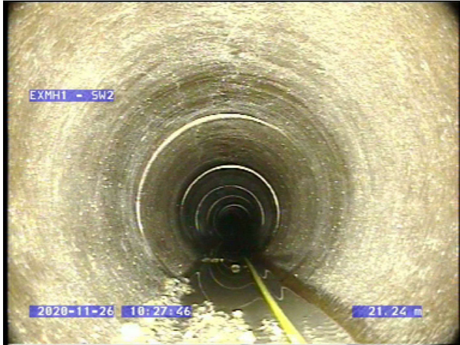
Photo: 5_5_37_A.jpg 21.25m, Settled deposits, coarse, 5% cross-sectional area loss, End
