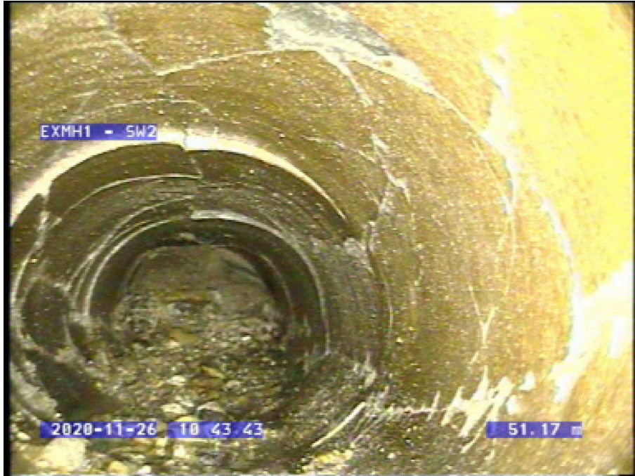
Photo: 5_5_57_A.jpg 51.55m, Collapsed drain/sewer
