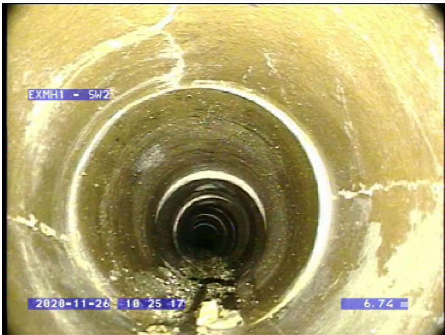
Photo: 5_5_31_A.jpg 6.8m, Cracks, multiple, from 12 to 12 o'clock, End
