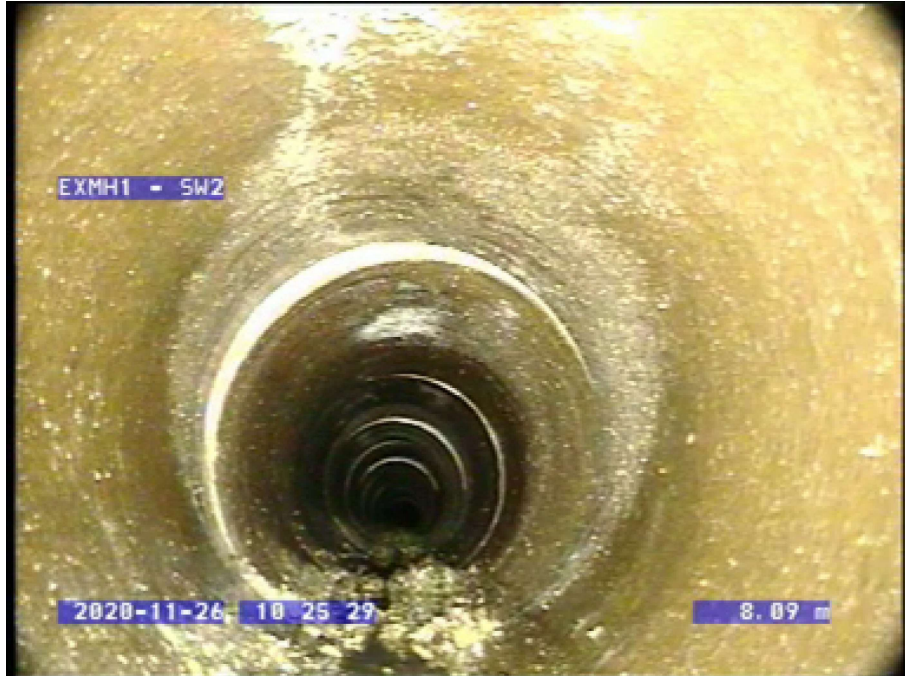
Photo: 5_5_32_A.jpg 8m, Settled deposits, coarse, 5% cross-sectional area loss, Start
