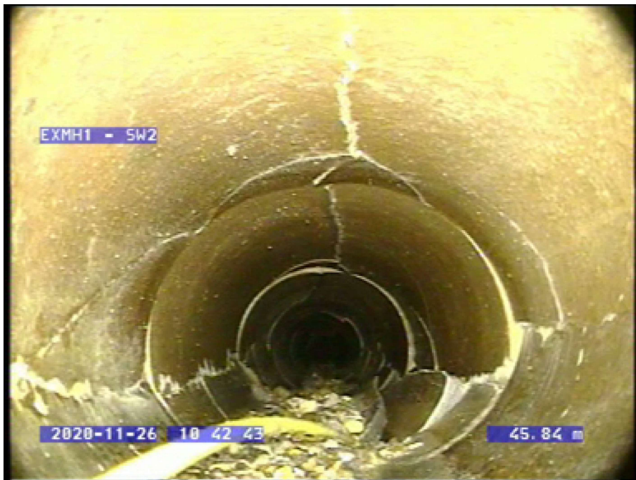
Photo: 5_5_52_A.jpg 45.8m, Settled deposits, coarse, 10% cross-sectional area loss
