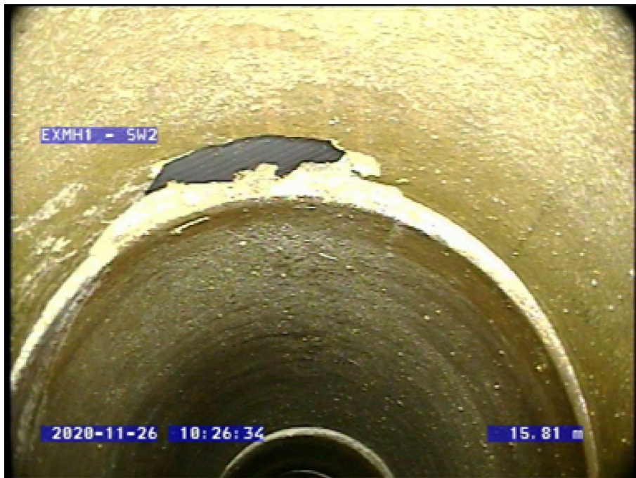
Photo: 5_5_33_A.jpg 15.8m, Hole in drain/sewer at joint, at 12 o'clock
