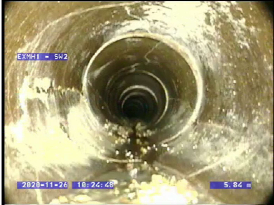
Photo: 5_5_30_A.jpg 5.8m, Cracks, multiple, from 12 to 12 o'clock, Start
