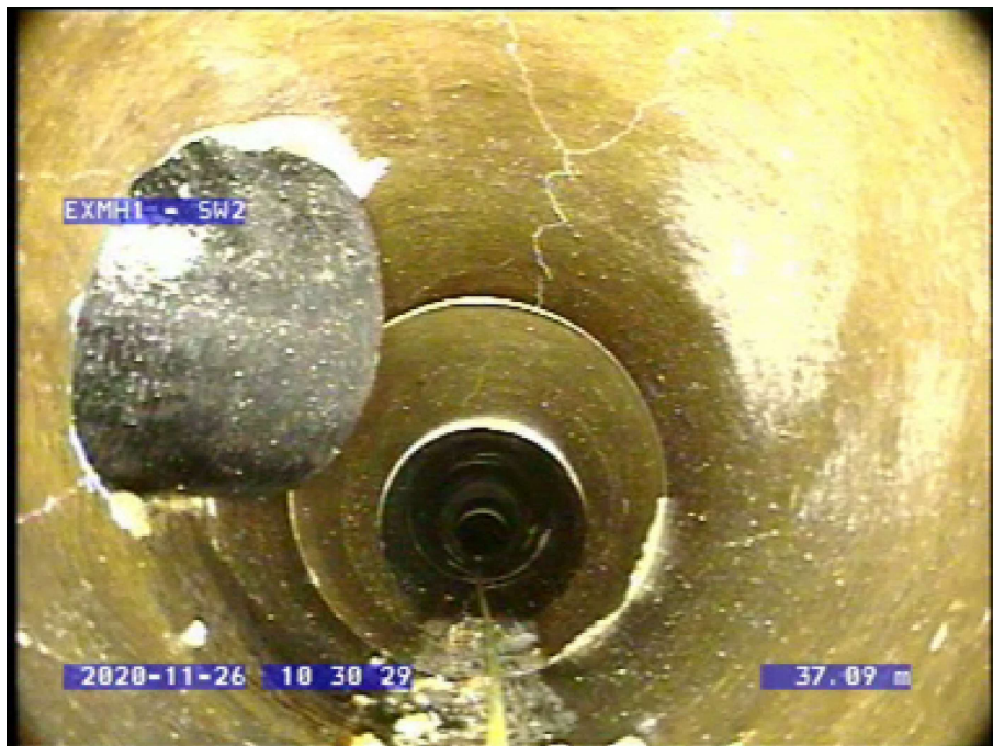
Photo: 5_5_43_A.jpg 37.1m, Connection defective, connecting pipe is damaged, at 9 o'clock, diameter 150mm, intrusion 15%
