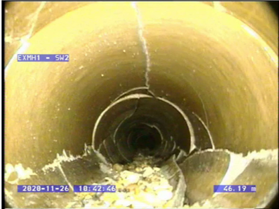
Photo: 5_5_54_A.jpg 46.2m, Broken pipe, from 12 to 12 o'clock, Start
