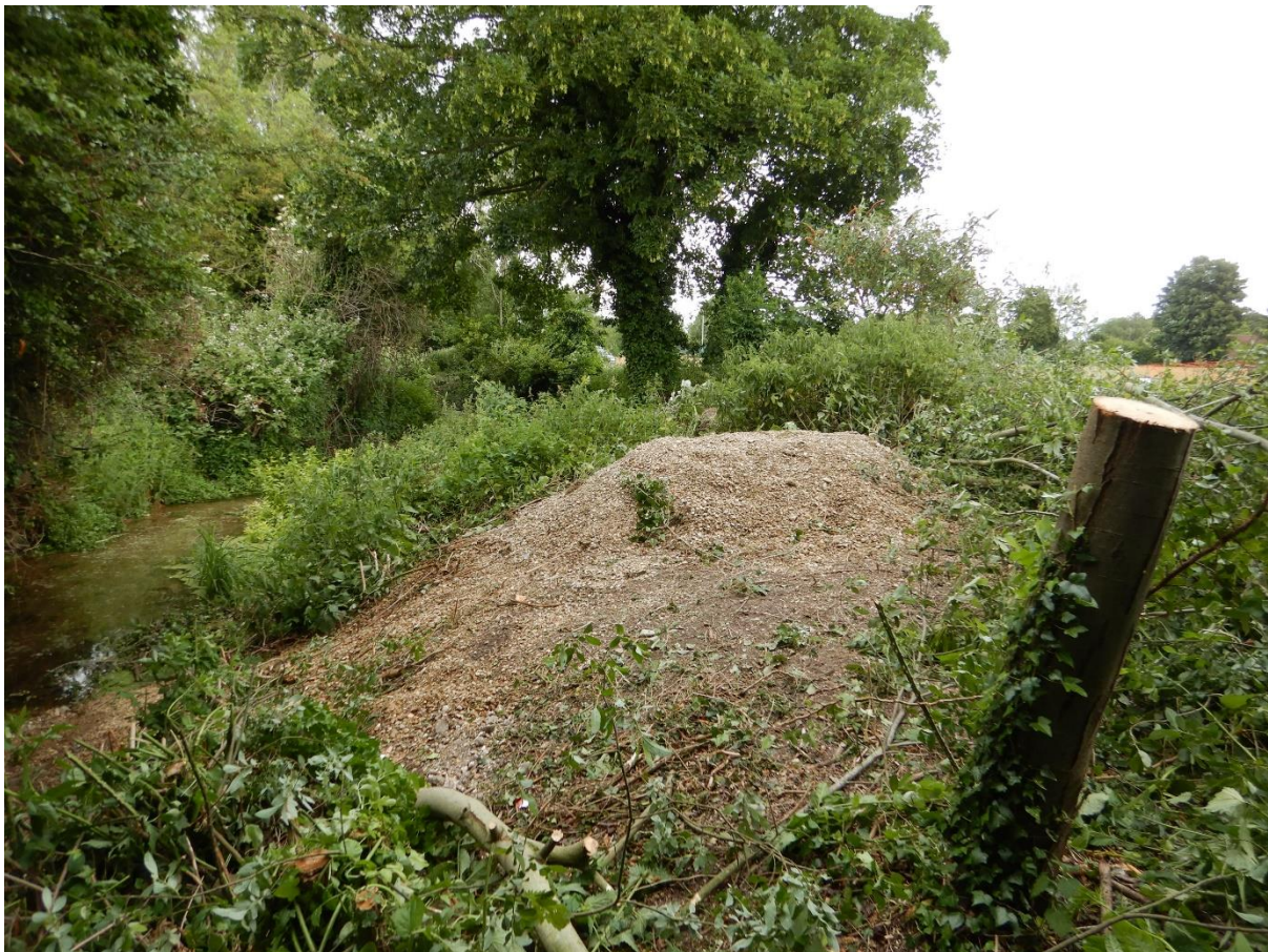
A small surplus of gravel and chalk has been left on site to allow for adjustments once the material settles. If the material requires moving, please do not hesitate to contact Rob Mungovan.
